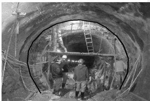
Fig. 3. Severe Tunnel squeezing seen at Chameliya Hydroelectric Project
